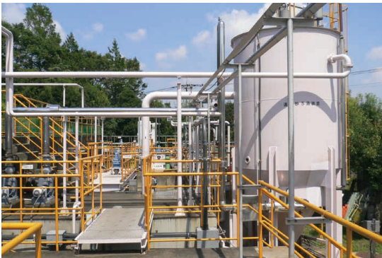
Wastewater treatment equipment (Itakura Facility)
