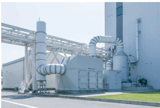
Deodorizing equipment (Itakura Facility)
