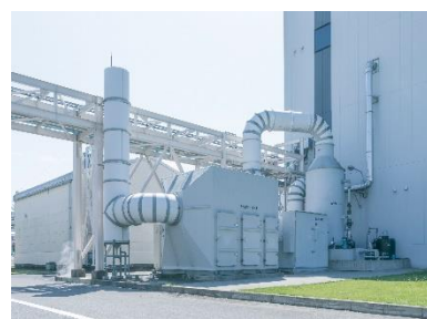
Deodorizing equipment (Itakura Facility)
