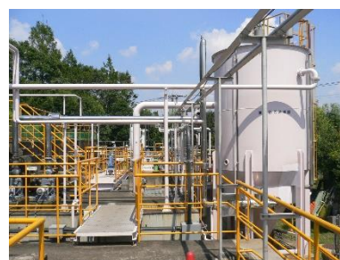
Wastewater treatment equipment (Itakura Facility)
